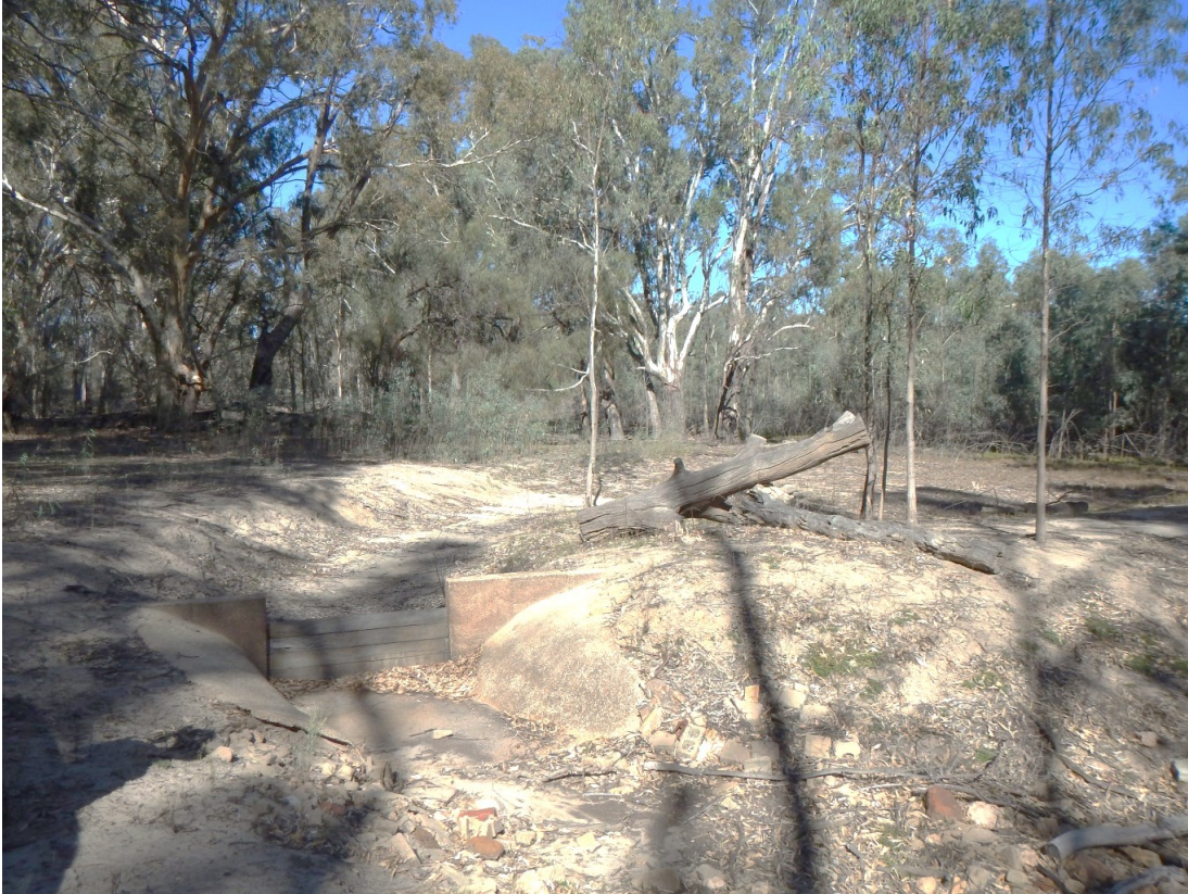
Figure 17. Photograph of a regulator structure still in use near the western end of Fishers Lagoon West
