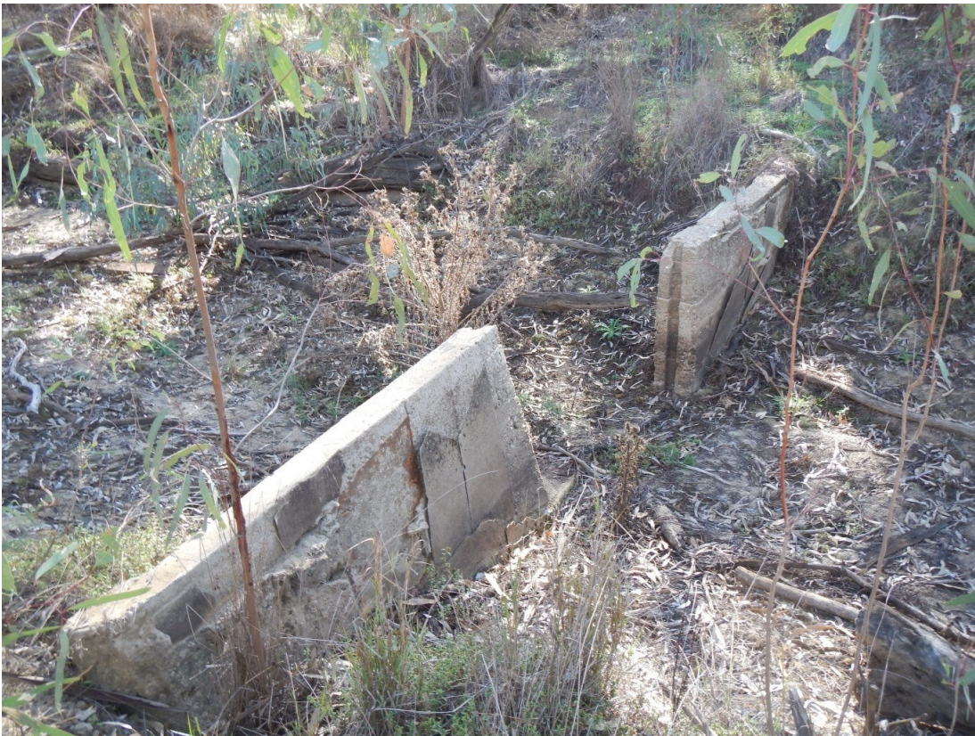
Figure 18. Photograph taken of a regulator structure in disrepair, this structure is located on the creek inlet to Central Fishers Lagoon
