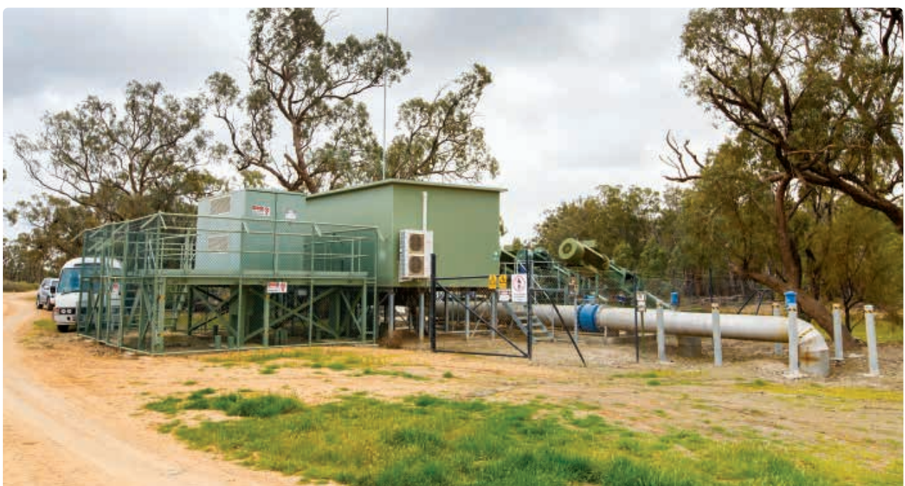
River Pumps at Robinvale.
